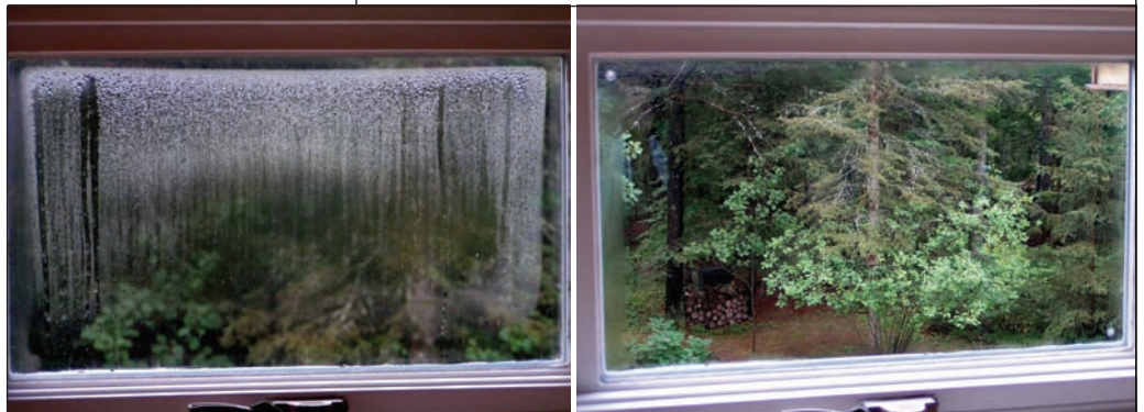
Before and after shots of a window that’s undergone the IG restoration process
